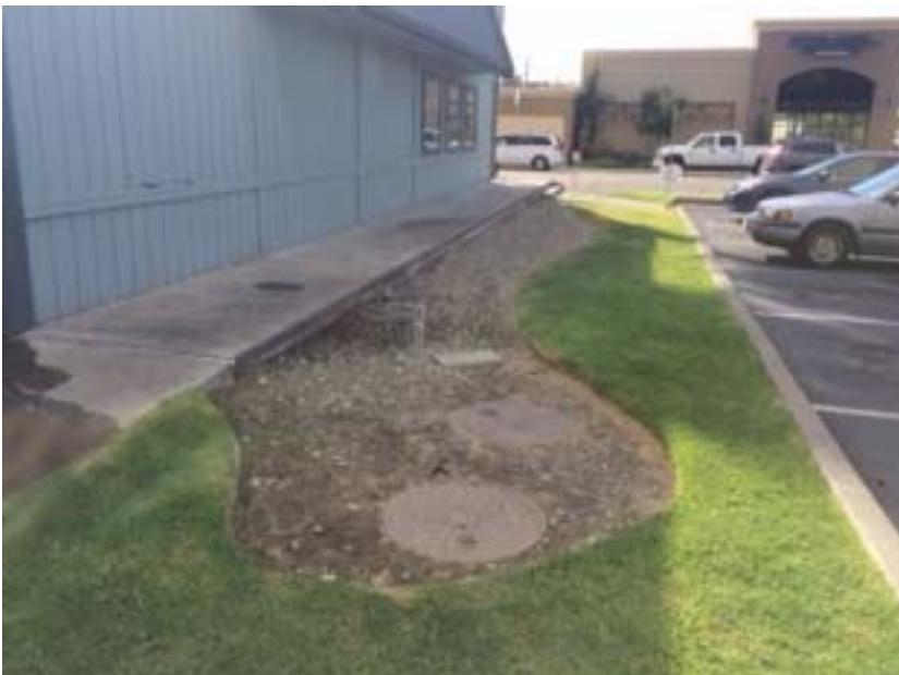
Grease interceptor in landscaping.
