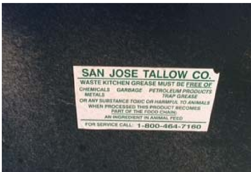
Interceptor in loading area for kitchen
