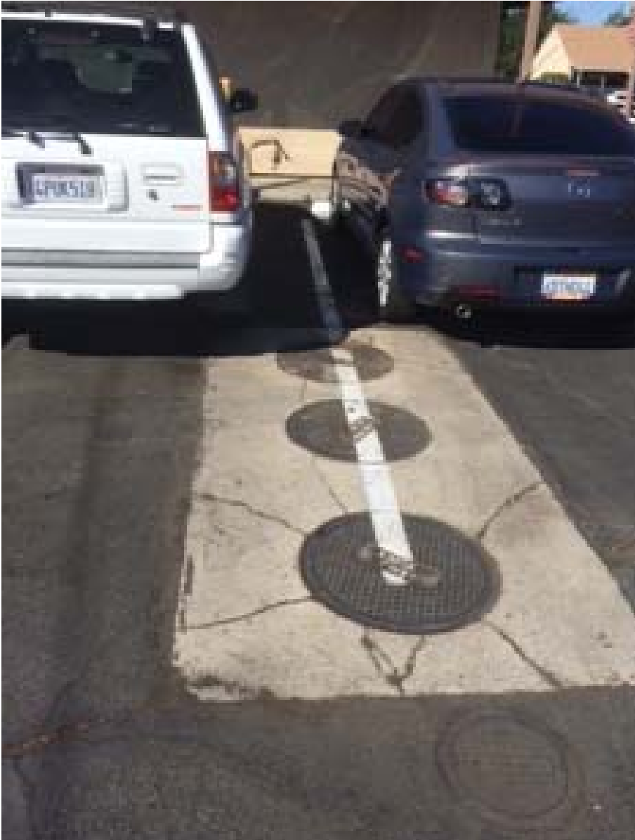
Triple cell interceptor on south side of building
