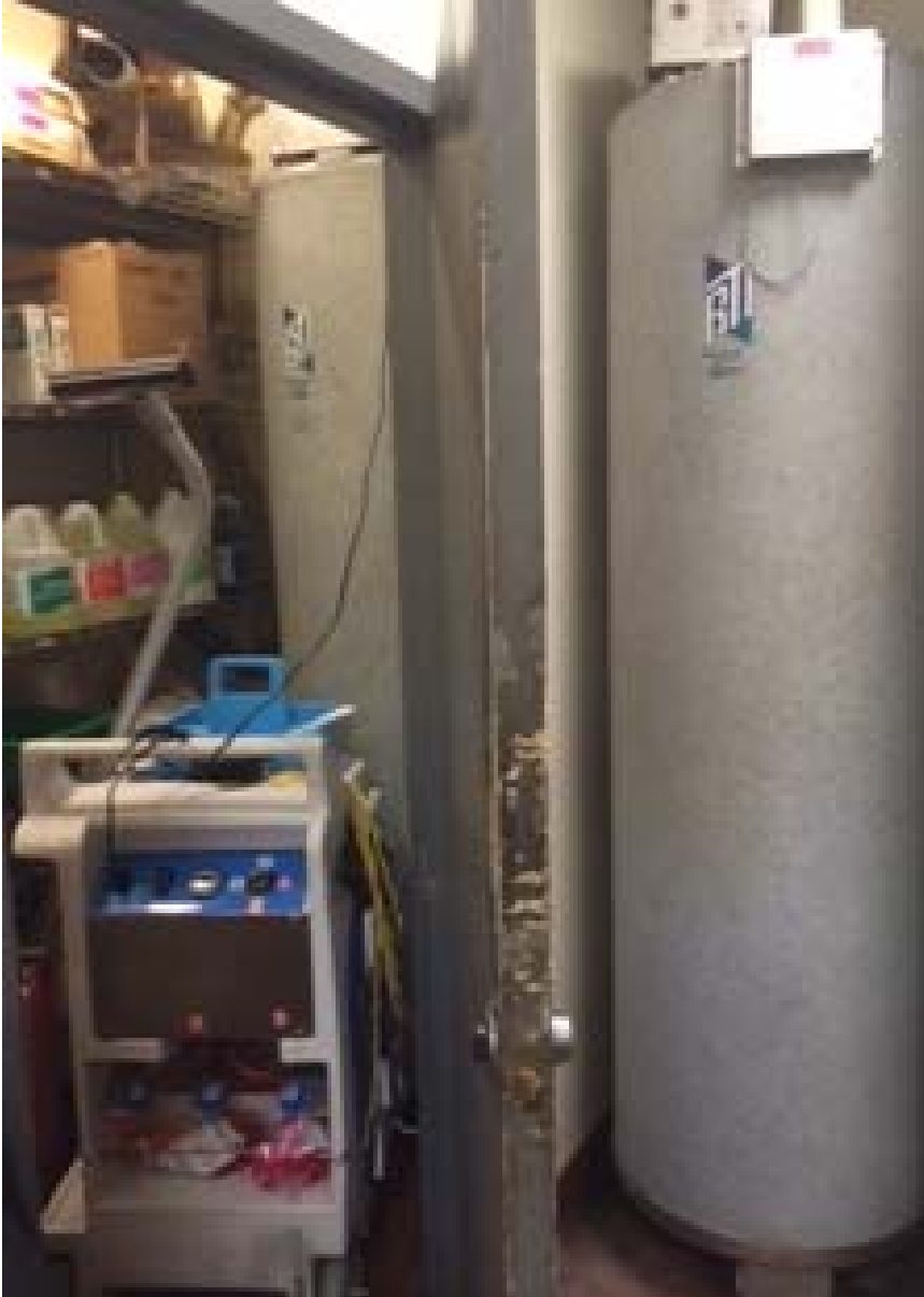
New and used oil storage
