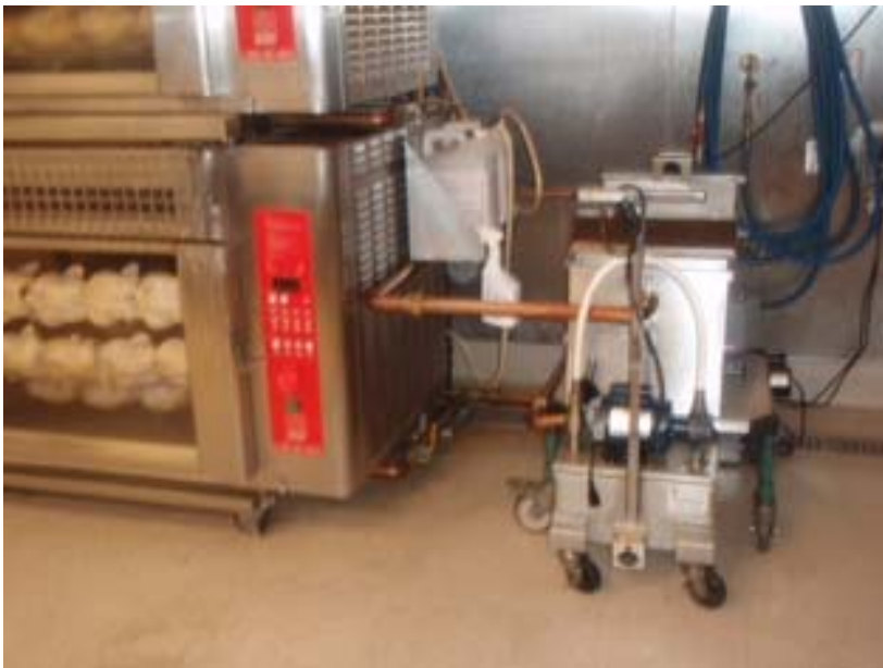
Costco kitchen and used oil storage.
