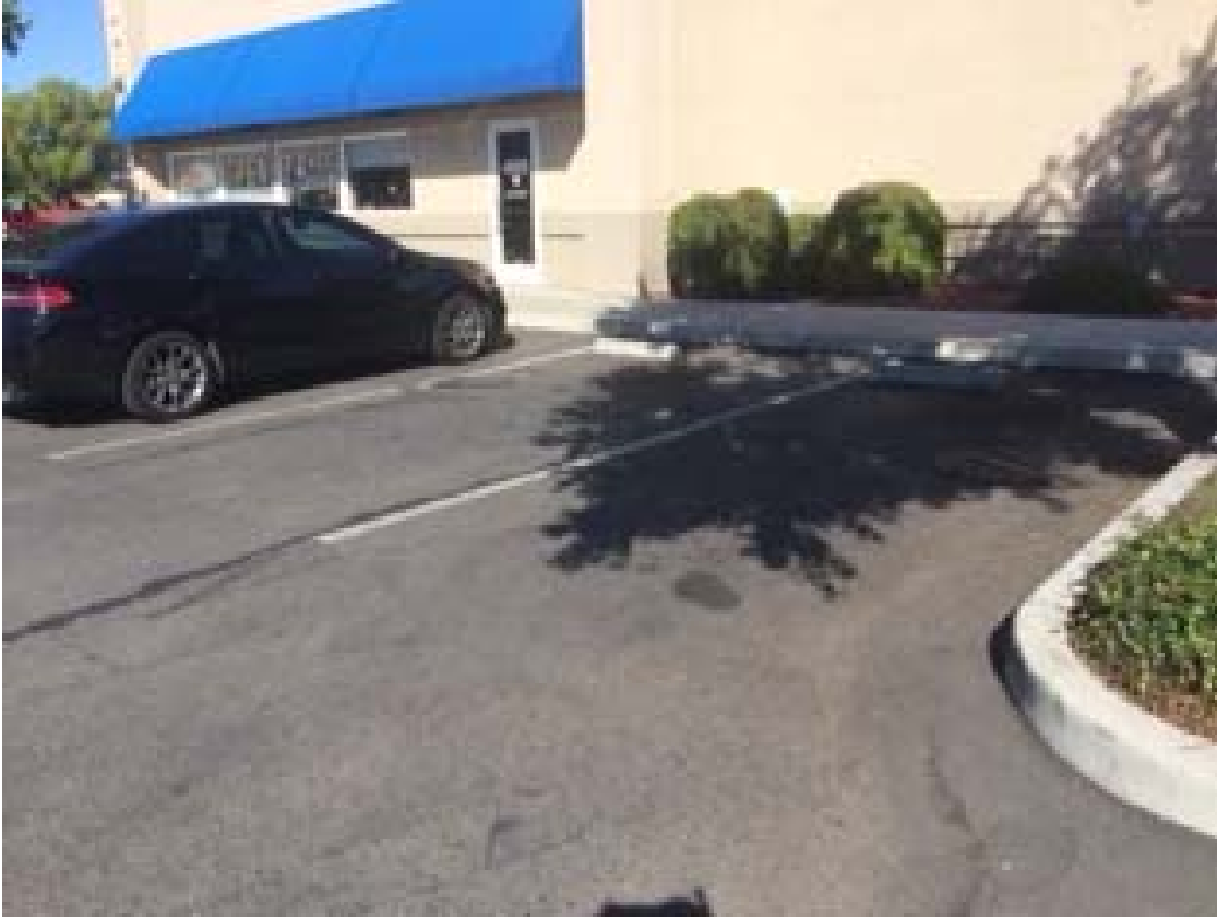
Interceptor in parking lot
