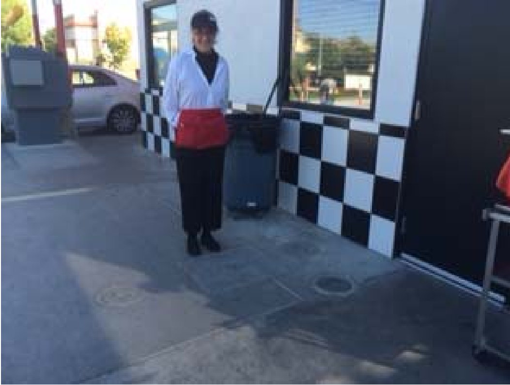
Small in the ground grease trap
