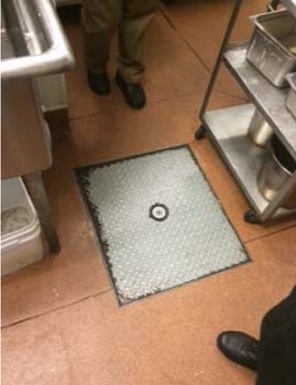
In the floor grease trap
