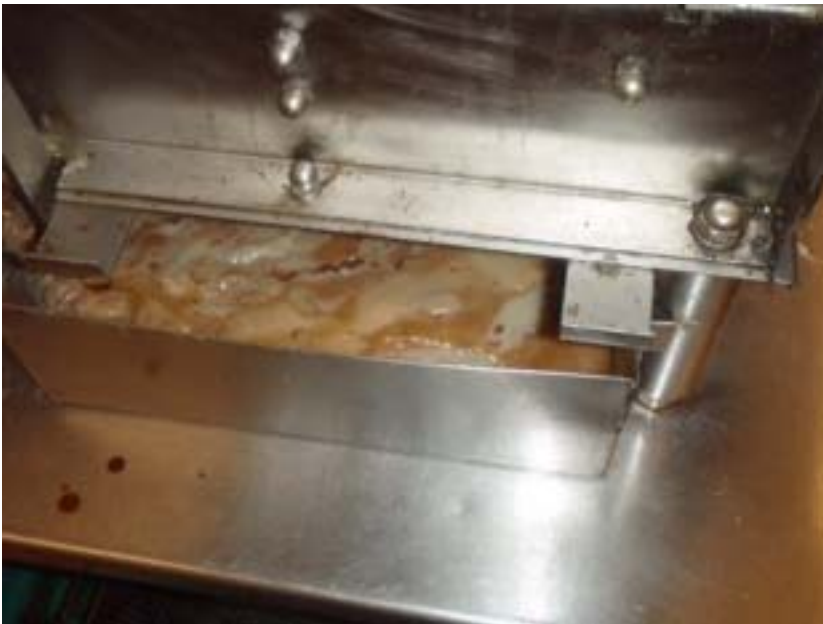
Grease captured in grill
