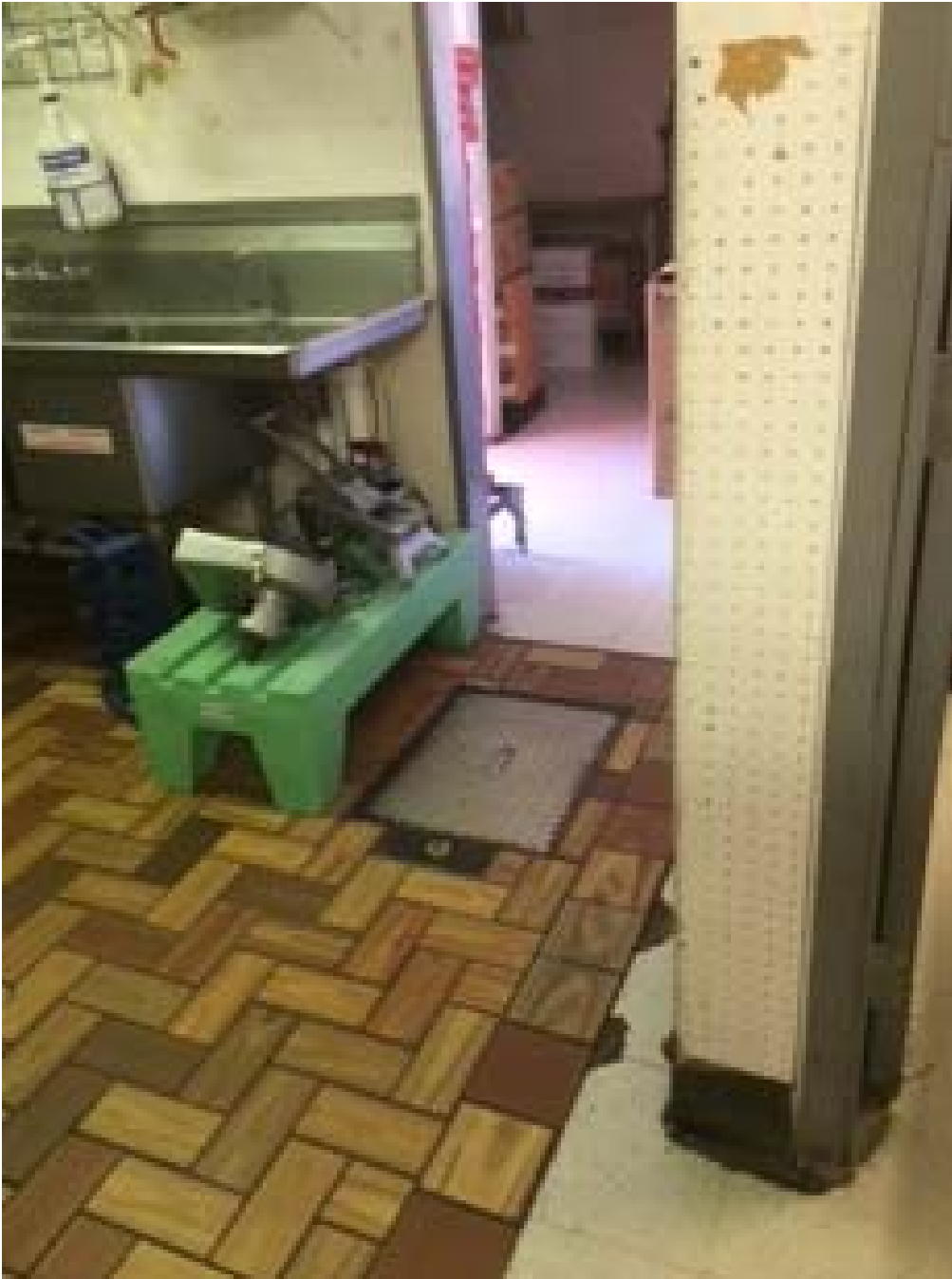
Small interceptor inside kitchen
