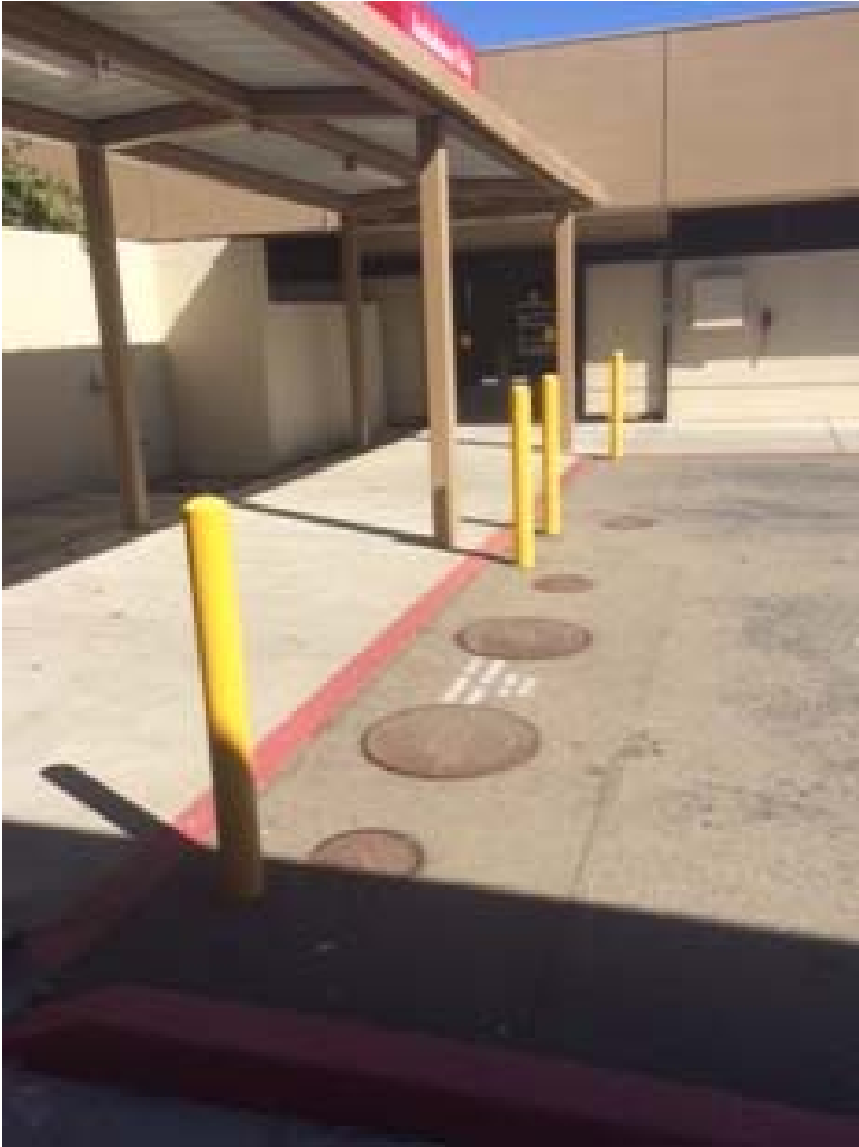
Interceptor in emergency entrance
