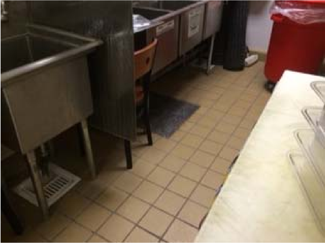
Under the sink grease trap
