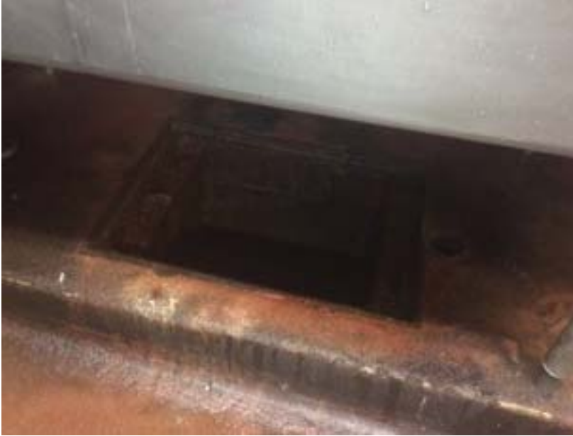
Small grease trap under sink. At the time of the picture the box was open for cleaning.
