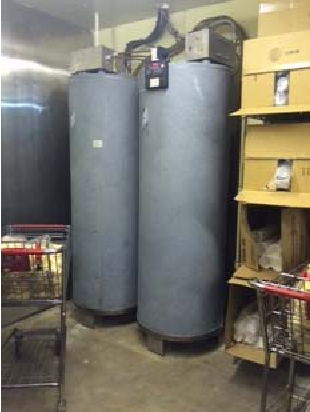
New and used oil storage, with telemetry
