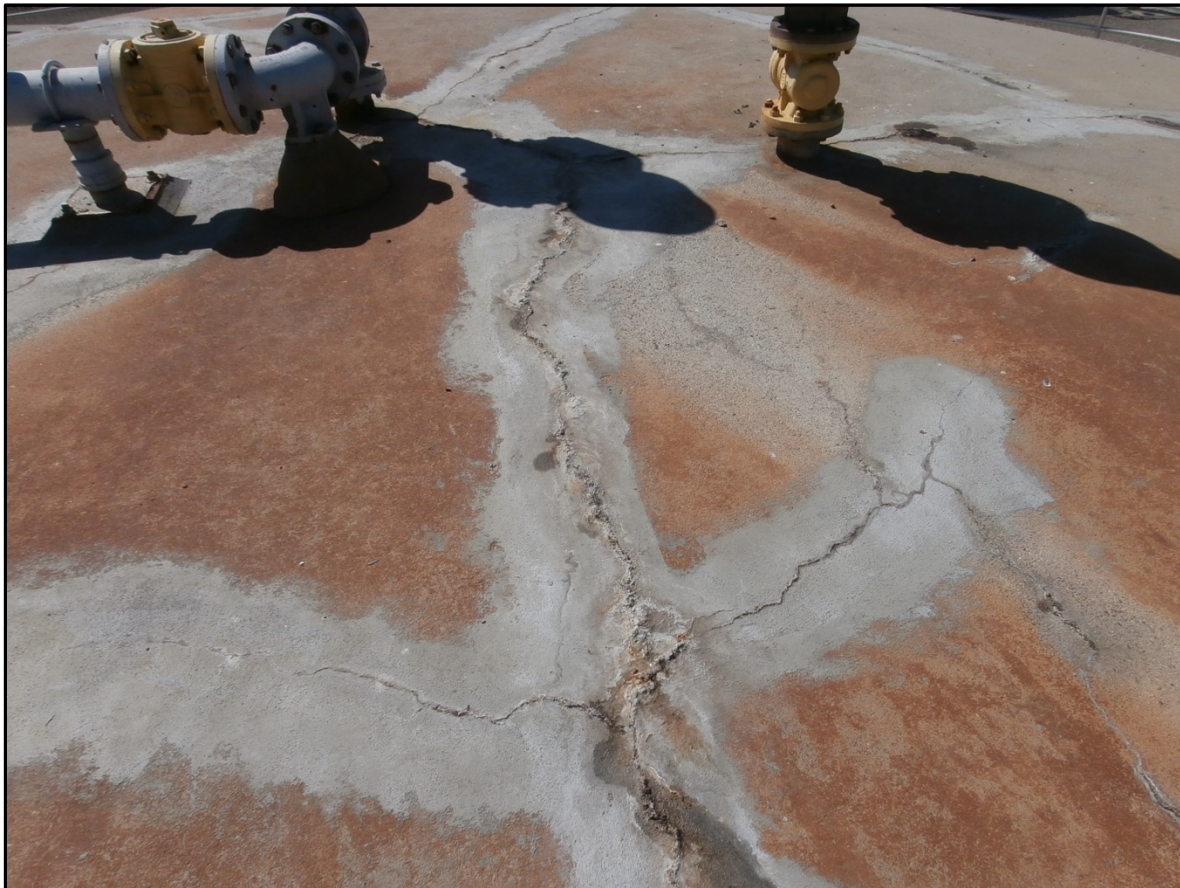
Figure 6.3-1, Typical Digester Dome Cracking
